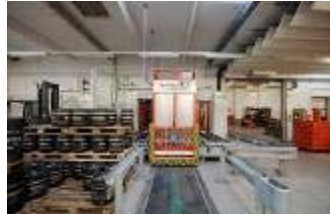
Image 4/5: Transfer car with inductive power supply at the disposal station of the conveyors in the production areas bottling and barreling.
